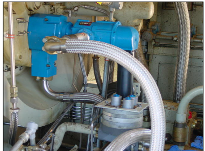
Figure 9. Air Starter Installation
